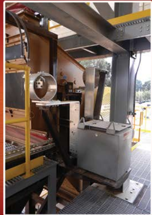
Screen heating installed on a Midwestern MEV®.
